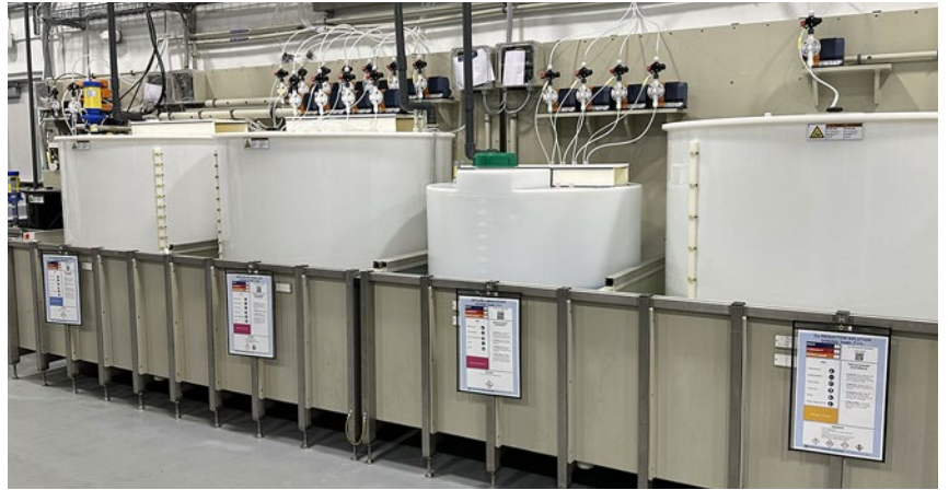
IPS automated dosing station at SEL's Idaho facility.
